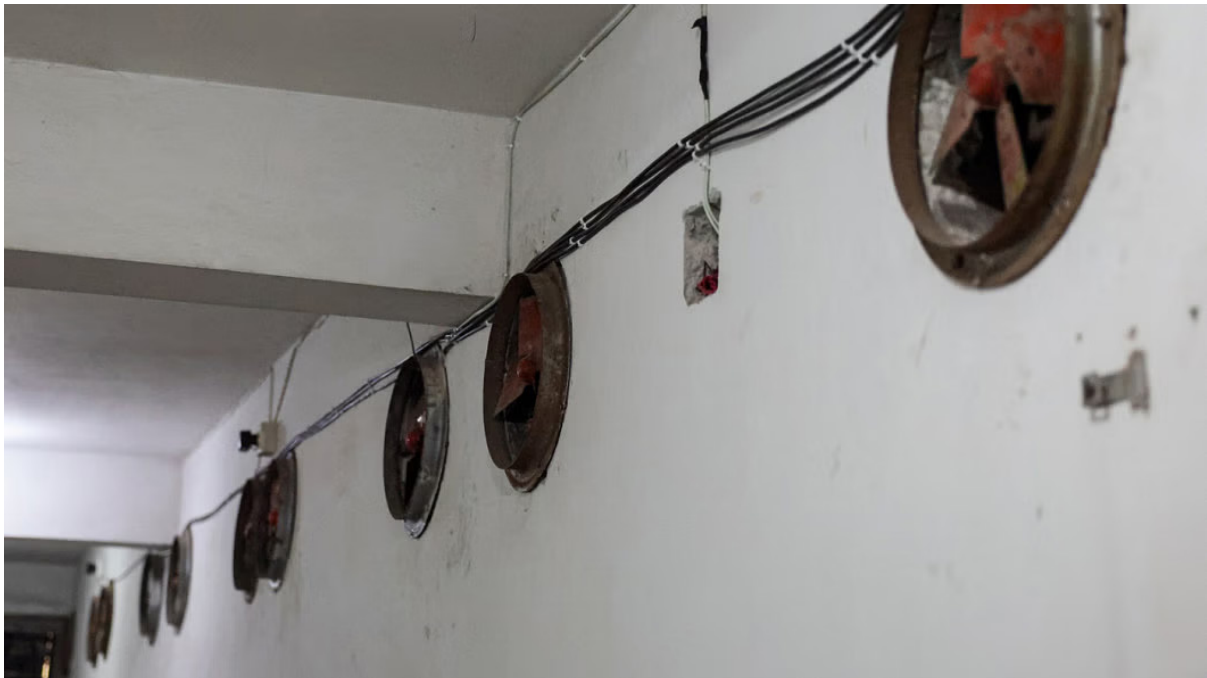
Figure 1b. Exhaust fan of Aynaghor (The Daily Star, 2025)
