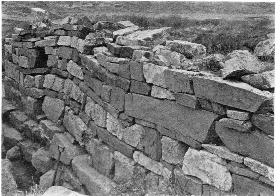
Fig. 19. Details of north wall of the church, showing the thick foundation and the wavy courses. Undir Höfða. Eastern Settlement No. 66. (From ROUSSELL, 1941, fig. 70).
