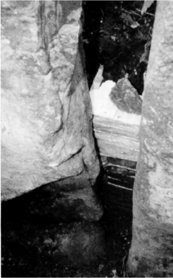
Fig. 8. In connection with the rebuilding of the dry walling under restoration work experiments were carried out with the use of birch bark, both between the original, re-used slabs and between newly shaped additions. Previous softening of the bark in water made handling easier. Passage grave north of Birkerød, 2000. Photo Torben Dehn.
