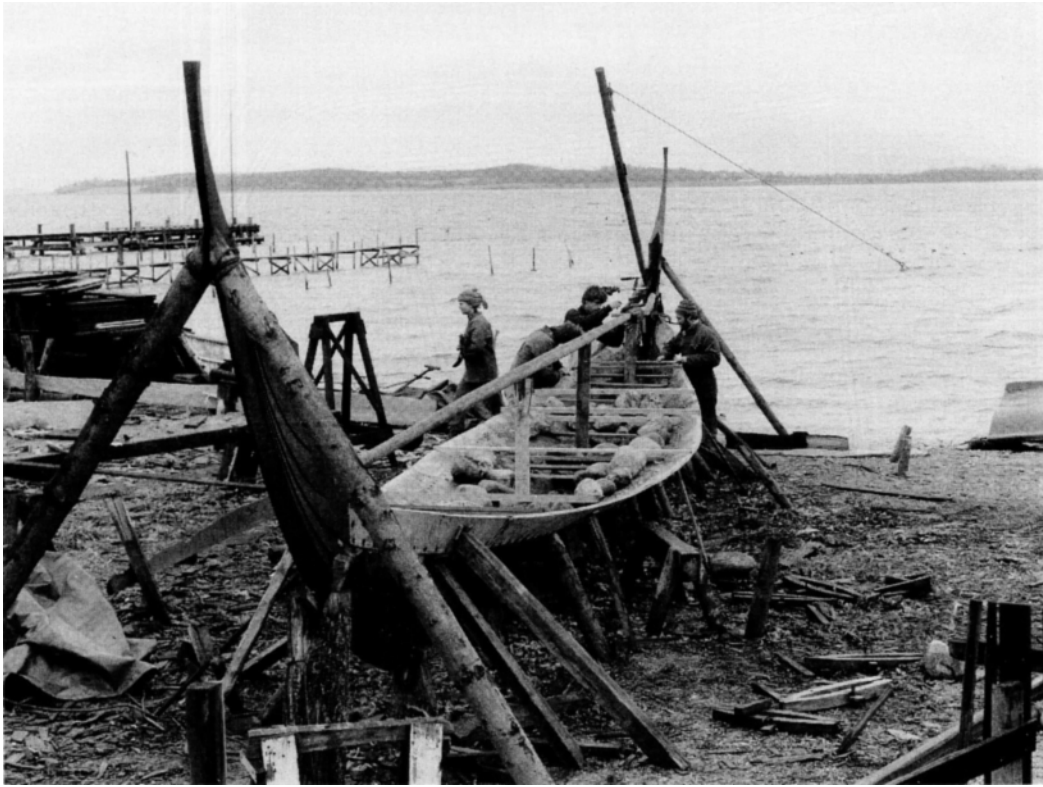
Fig. 5. ROAR EGE under construction in Roskilde in October 1983. The bottom planks have been fitted and are held in position by sticks from below and stones from above.
