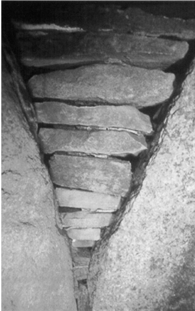
Fig. 2. Dry walling with birch bark in situ in Maglehøj. In the uppermost course no bark can be seen but in the second to the fifth course from the top the fold is preserved to varying degrees. In the sixth course there is bark but the fold is missing. The section shown is 50 cm high. Photo Torben Dehn.
