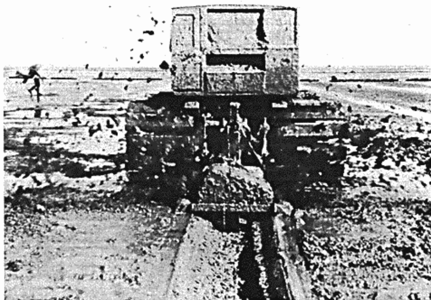
Fig. 6. The ditching-plough, drawn by a caterpillar-tractor. The ditch is dug so as to have an obliquely declining border; the material is thrown to both sides, forming a slightly curved field ridge. B. Jakobsen, Kr. M. Jensen & Niels Nielsen, Medd. f. Skall.-Lab. XV.
