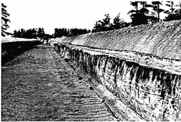
Fig. 2. View along the gas pipe-line trench. Before trenching, the top soil has been removed and the lower part of a podzol is visible. The face in the trench shows a cover sand deposit. The visible part of the face is approximately 1.7 meters deep.
