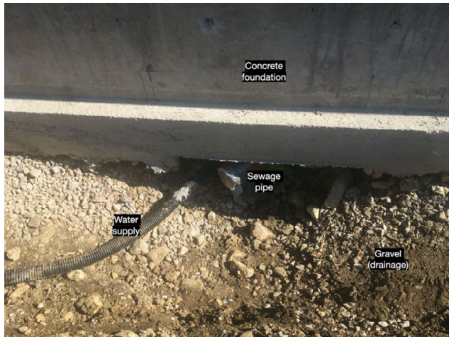
Figure 6: The sewage pipe leading out of the concrete foundation, to be connected to the main sewage system
