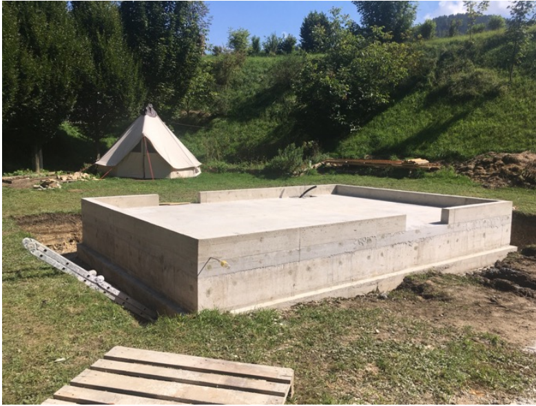
Figure 1. Photograph of the foundations forming part of Neubauer's 3000m 2 prototype. Image credit: Ruth Neubauer.
